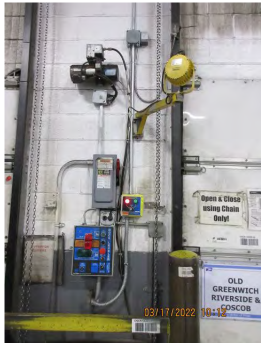
Existing Red/Green Light Controls, Left side of DOOR 22
