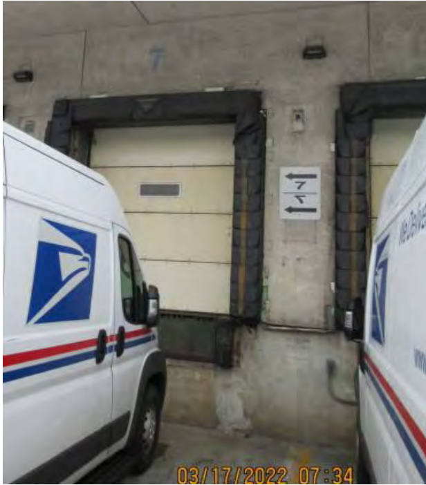
DOOR 7 Install Kelley Dock Communication System
