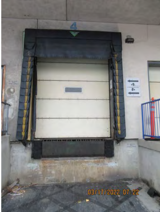
DOOR 4 Install Kelley Dock Communication System
