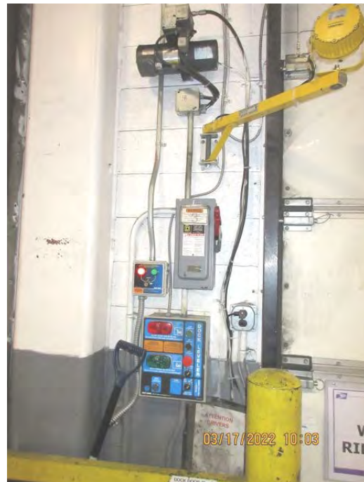
Existing Red/Green Light Controls, Left side of DOOR 19
