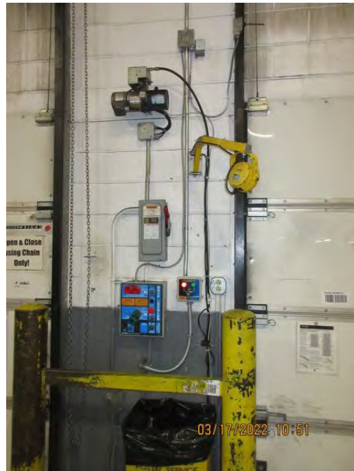
Existing Red/Green Light Controls, Left side of DOOR 31
