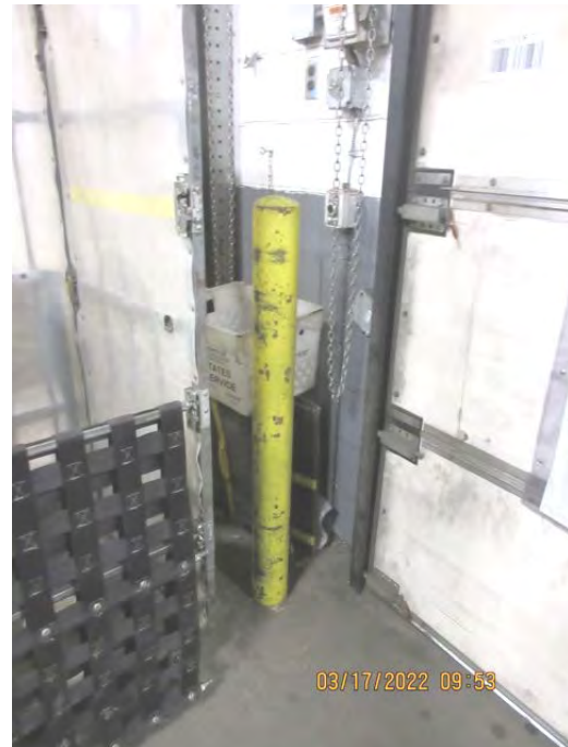
Dock Leveler Controls, Left side of DOOR 17
