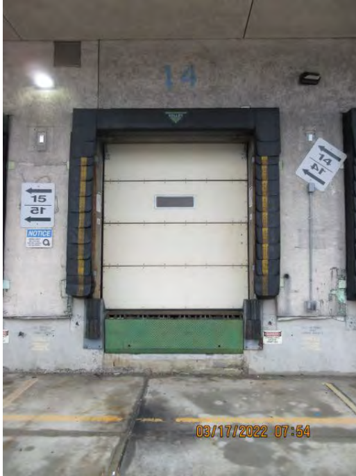
DOOR 14 Install Kelley Dock Communication System
