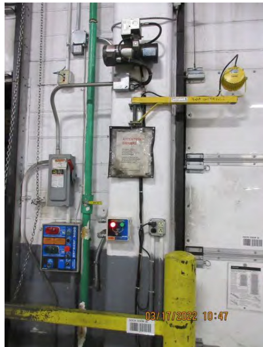
Existing Red/Green Light Controls, Left side of DOOR 30
