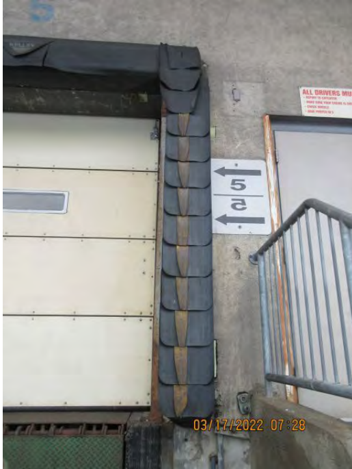
DOOR 5 Install Kelley Dock Communication System
