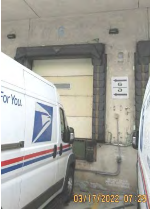
DOOR 6 Install Kelley Dock Communication System
