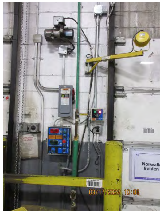
Existing Red/Green Light Controls, Left side of DOOR 20
