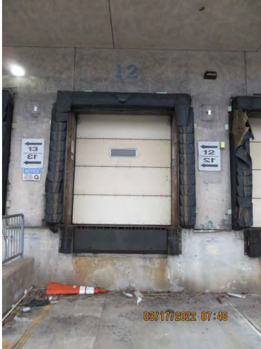
DOOR 12 Install Kelley Dock Communication System
