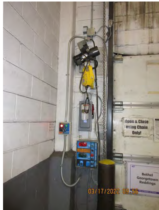
Existing Red/Green Light Controls, Left side of DOOR 18
