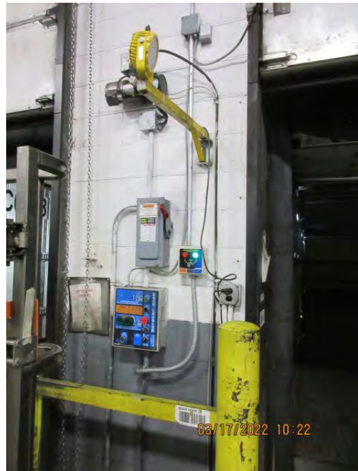
Existing Red/Green Light Controls, Left side of DOOR 24
