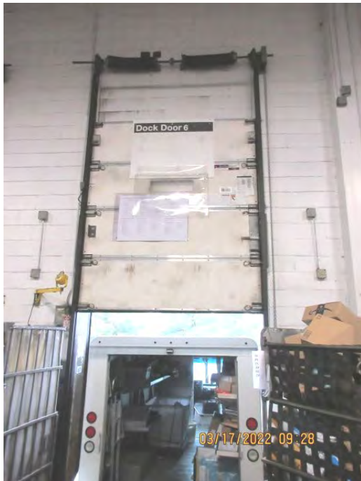
Dock Leveler Controls, Left side of DOOR 6
