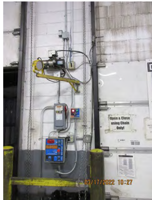
Existing Red/Green Light Controls, Left side of DOOR 25
