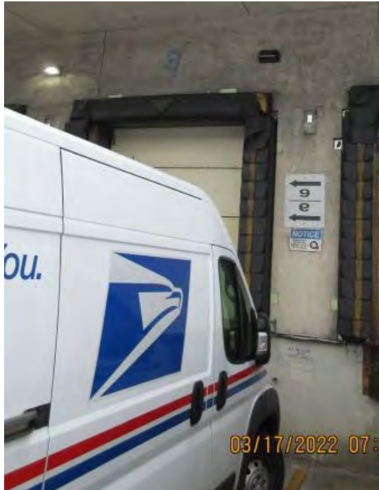
DOOR 9 Install Kelley Dock Communication System
