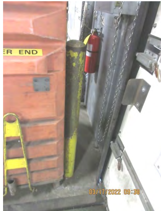
Dock Leveler Controls, Left side of DOOR 10
