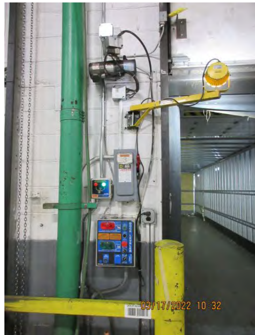
Existing Red/Green Light Controls, Left side of DOOR 27
