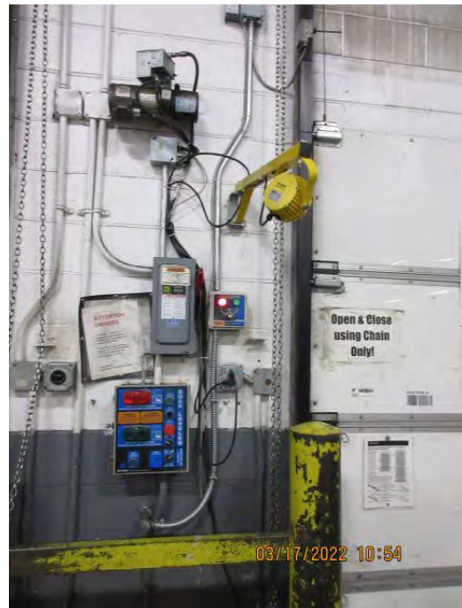
Existing Red/Green Light Controls, Left side of DOOR 32
