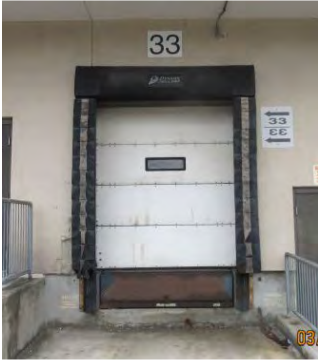
DOOR 33 Install Kelley Dock Communication System
