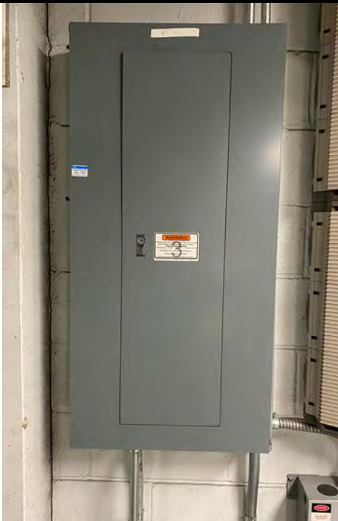
DOORS 4-7 Panel RPM.5-2.7 Add New 1 Pole 20A Circuit Breaker (1 for every 4 Doors)
