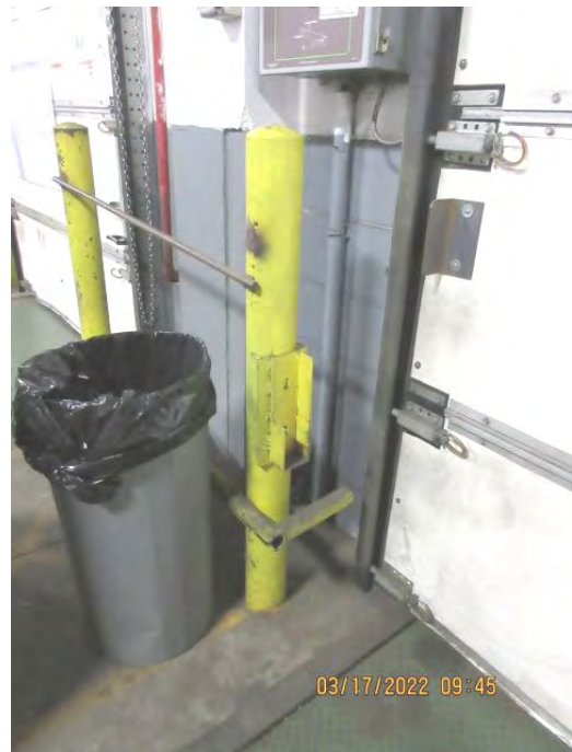
Dock Leveler Controls, Left side of DOOR 13
