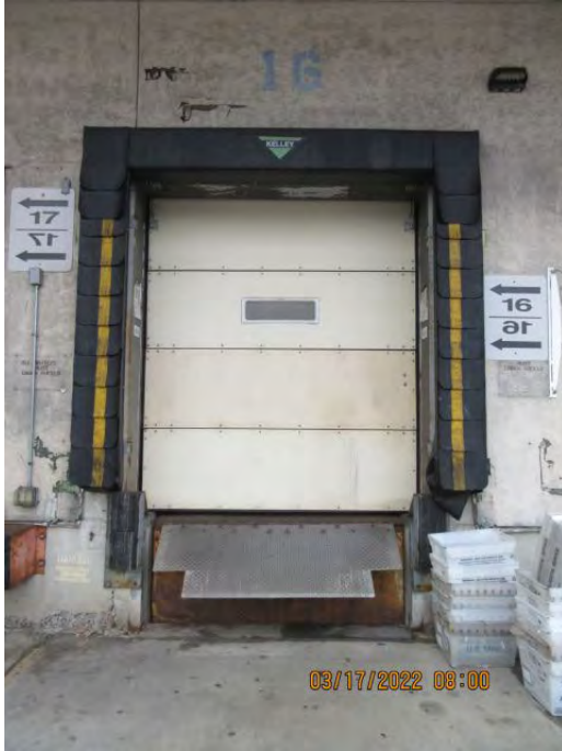
DOOR 16 Install Kelley Dock Communication System
