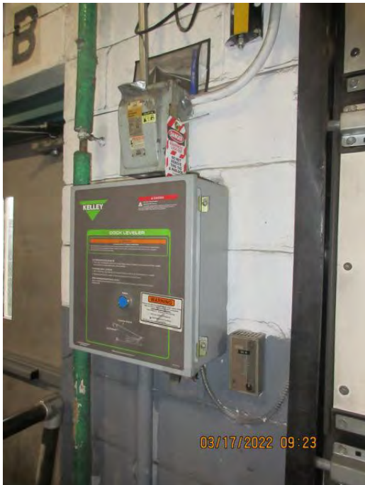
Dock Leveler Controls, Left side of DOOR 5
