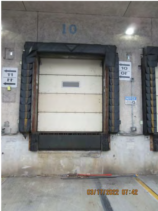
DOOR 10 Install Kelley Dock Communication System
